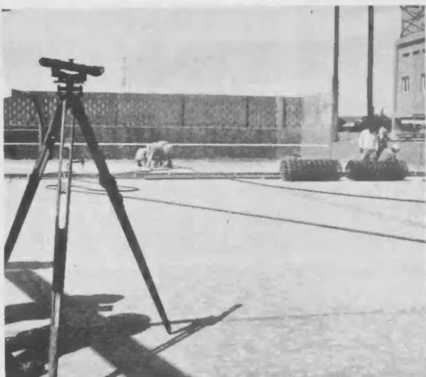
TO INSURE level placement of forms and screeds, a theodolite serves as constant reference. Into the forms, complete with reinforcing rods, is poured the concrete, about 36 cubic yards at a time.
